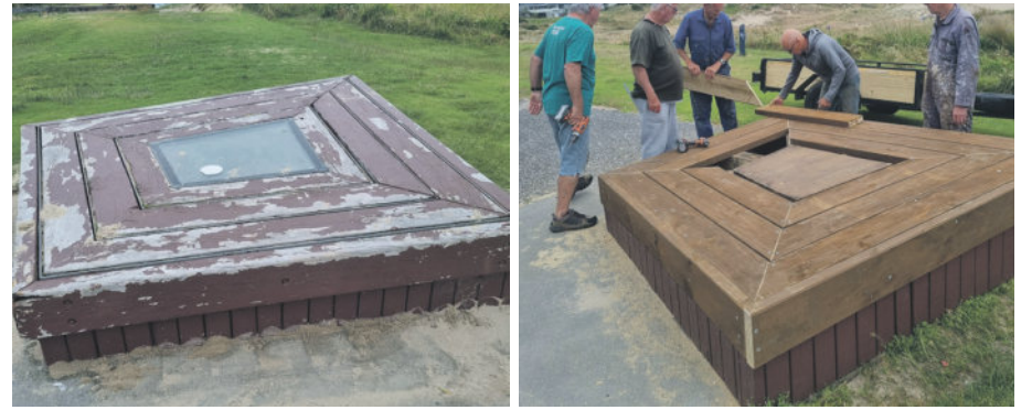
The Menzshed are currently upgrading seats and viewing platforms in Hunt Rd. The photos above are of the viewing platform before and a work in progress.
